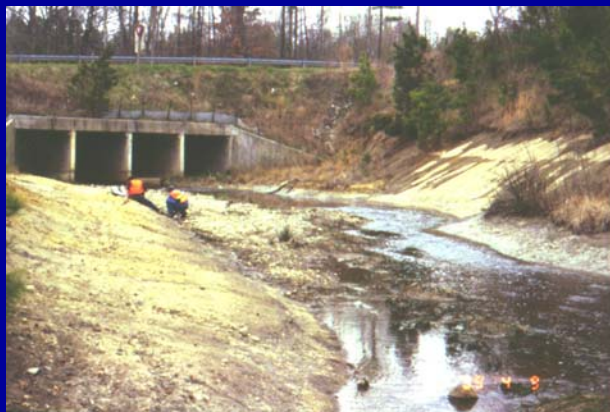
Chesterfield County: Proctor's Creek was redirected to this excavated channel during road construction.
